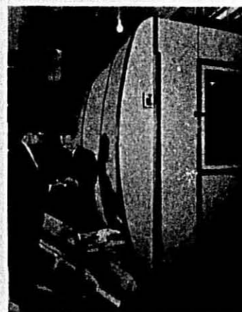
H. Geddes Stanway, executive vice-president of the Skinner Manufacturing Company of Omaha, and William Berger, Buhler Brothers sales engineer, inspect the product discharged from the new Buhler short goods preliminary dryer installed at Skinner.
